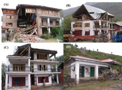
Fig -1: Damage observed in hybrid buildings in the Kashmir earthquake, 2005 (photo courtesy: CVR Murty)
