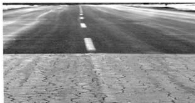
Fig -4: Rubberised bitumen chip seal applied to badly cracked pavement
