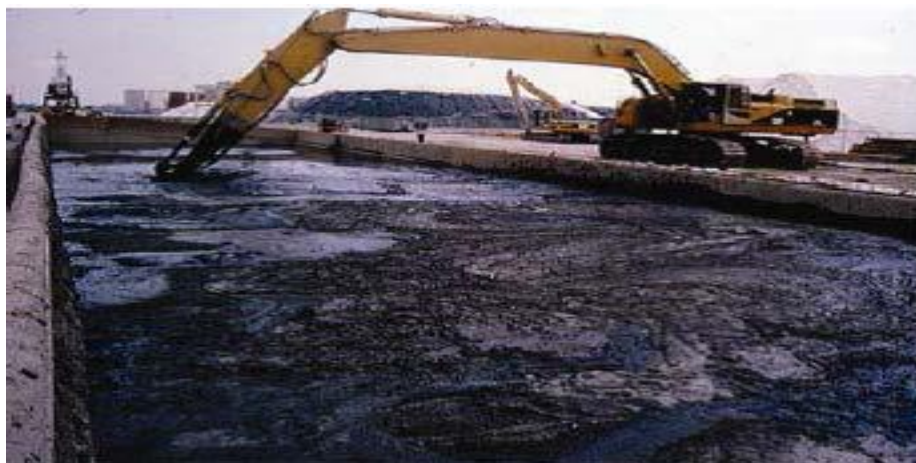
Ex-situ for on-site use stabilization (mixing in place of contaminated dredged materials)
