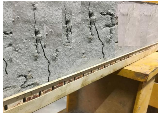
Fig.20: Crack patterns in the beam
