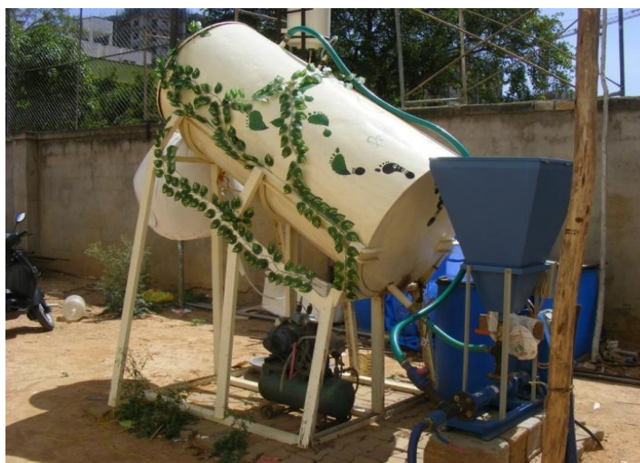
Fig 3- Picture of Biogas plant
