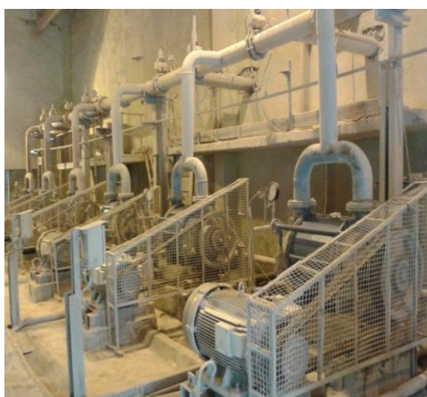
Image:- Vacuum Pumps in Ash Handling Plant.
