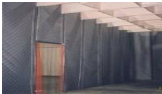
Figure 3: Wall Panels to reduce Noise
