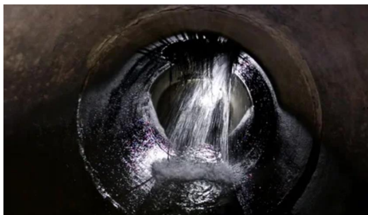
Figure 2: Pipe leakage in a wastewater pipe
