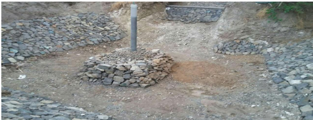
Image No. 4 – Filtration Chamber
