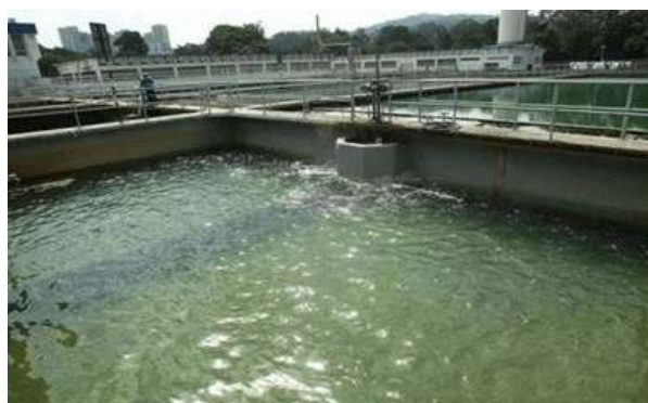
Image 1. Sewage treatment plant.
