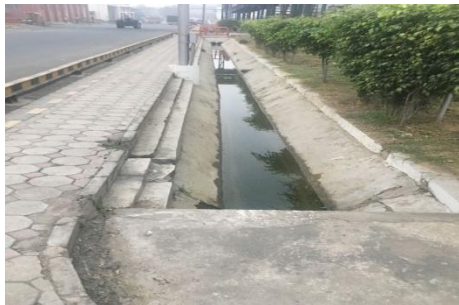
Image 1. These small drains spread in all over in plant help for passing waste and harvesting water.
