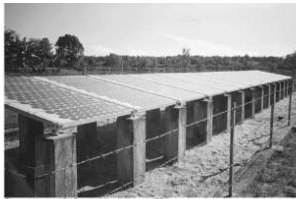
Figure 1. Array of PV Panels.
