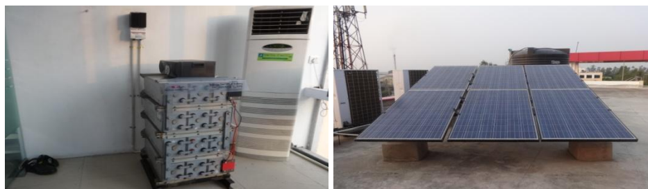
Figure 5.4: Solar Power system
