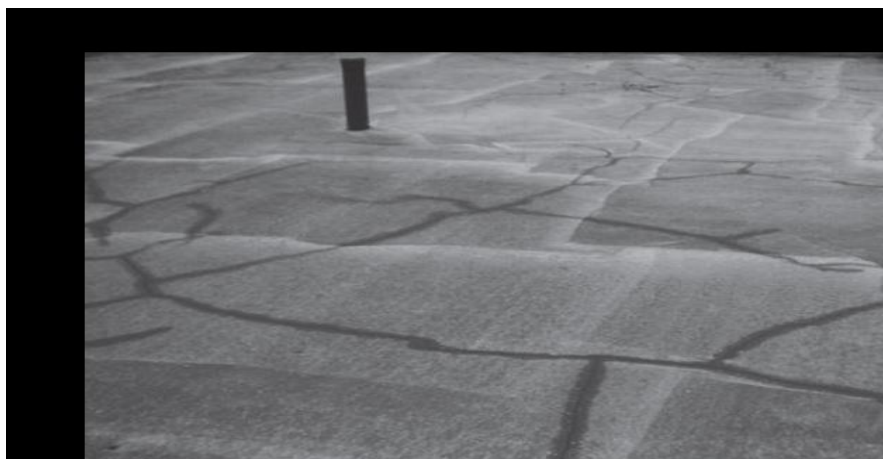
Fig.1 Plastic shrinkage cracking at concrete surface
