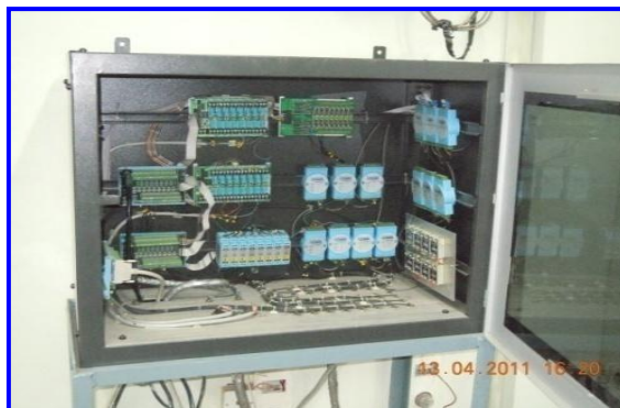
Fig 5: control panel for SO concentration, pressure measurement
